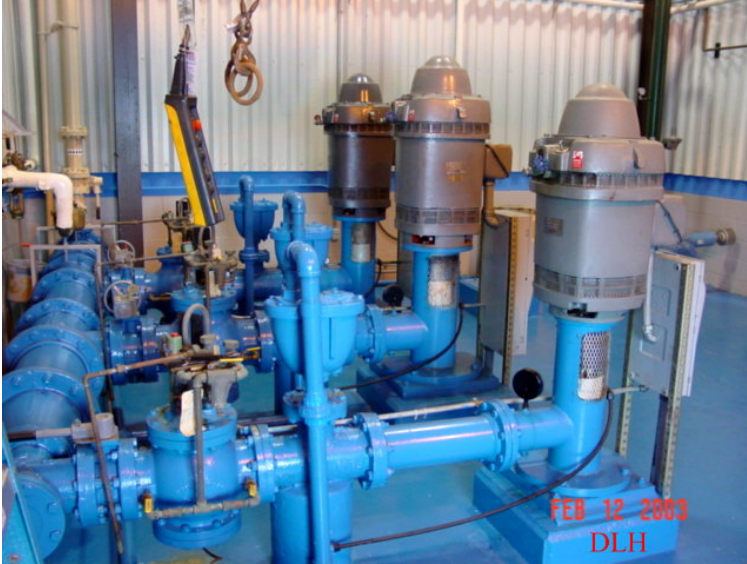
Figure 2. Vertical turbine pumps in clear well.
